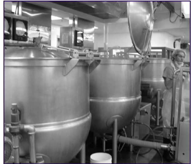
Cook-chill cooking and bagging system.
