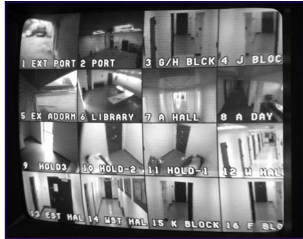
Black-and-white CCTV camera monitor with multiple views shown simultaneously.
