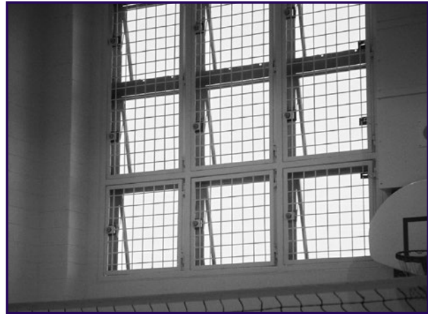
Secured windows in an indoor recreation yard. Note that these windows open for air circulation but have security mesh to prevent penetration. (Photograph courtesy of Voorhis Robertson Justice Services.)
