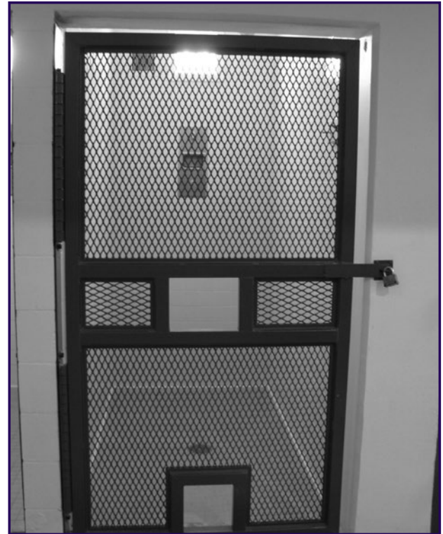
A secured shower in an administrative segregation unit. Note the ports used to remove restraints.
