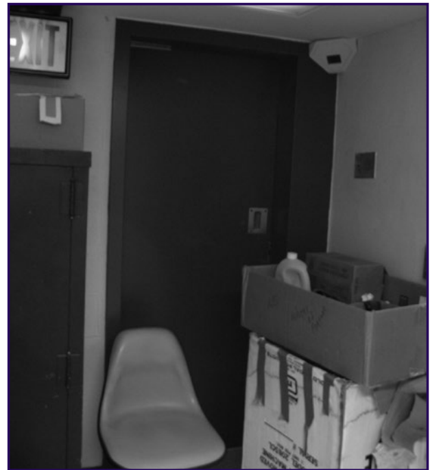
Fire exit blocked with stored items in violation of fire codes. (Photograph courtesy of Jim Rowenhorst.)
